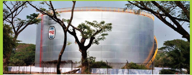
Padma Oil Company Ltd. Automatic Fire Hydrant & Foam System
