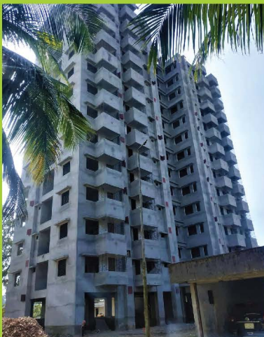
Bangladesh Air Force-BAF. Automatic Fire Hydrant System & Fire Detection & Alarm System.
